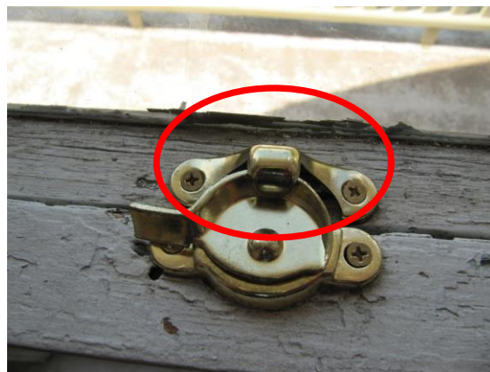
Shown locked; note lock "hood" over arc.
